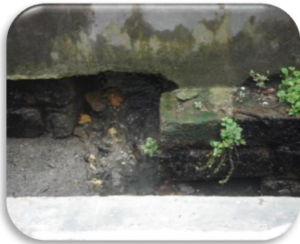
Fig: Human waste discharge to drain
