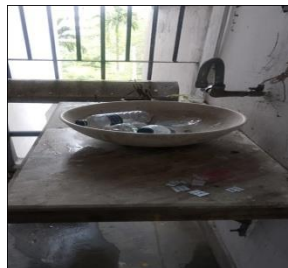
Fig: Hand wash facilities are unuseable
