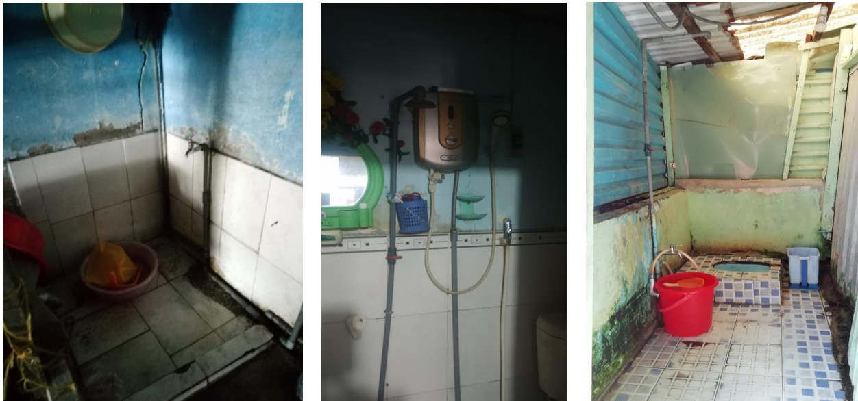
Figure 3: a) Safe drinking water supply for the marginal b) Installed water heating system & Hygiene tools available c) Decent Toilet with safe water supply, adequate sanitation and Hygiene facilities
