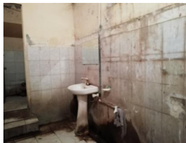
Fig: Unhygienic hand wash facility
