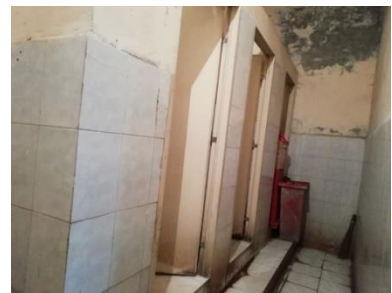
Fig: One toilet is blocked
